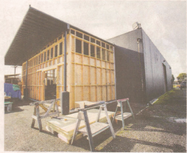
The Coastal Repertory Theatre in Half Moon Bay is addressing a problem for many community groups — storage. It is building on to its existing location on Main Street.
